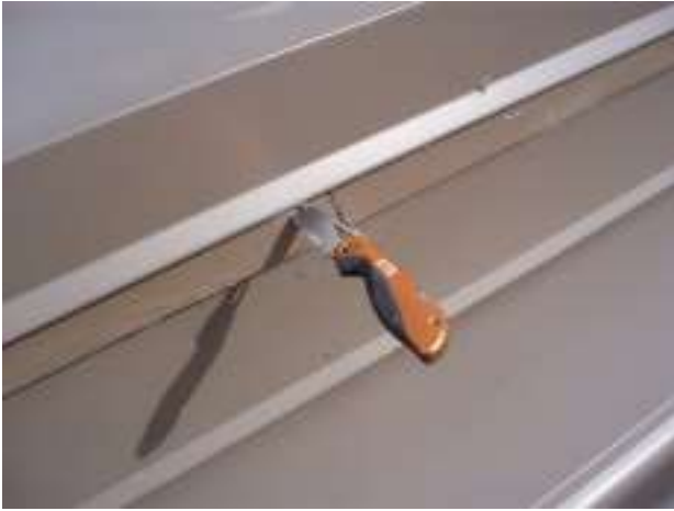
37. The fascia board where the garage roof steps up by the master bedroom is decayed & I was able to push my pocket knife into it.
