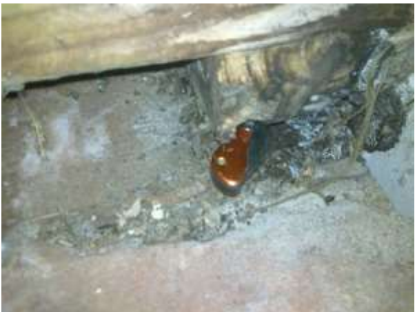
39. This is a severely decayed bearer which sits on top of a masonry foundation wall. I met no resistance at all when I pushed my knife into this.
