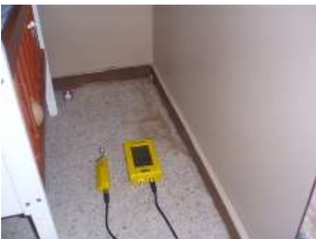
24. Water staining is clearly visible on the carpet in the SW corner of the rumpus.
