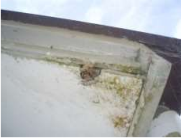
21. This is the SW corner of the eaves. This definitely leaks.
