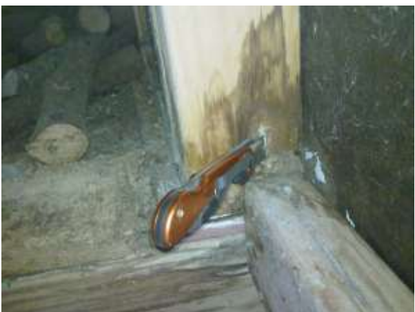
40. A badly decayed jack stud.
