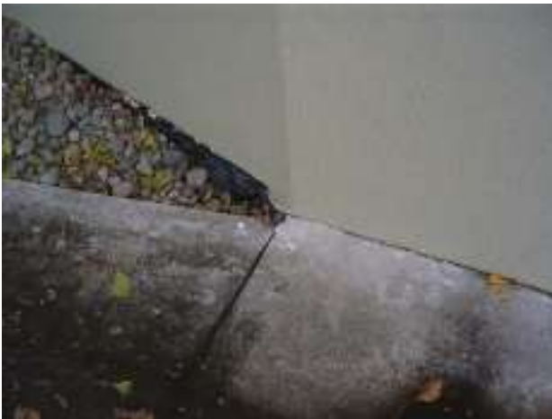
22. The South wall of the garage & rumpus room has cladding which extends below the adjacent ground level. This is a very bad detail which inevitably leads to trapped moisture & decay.
