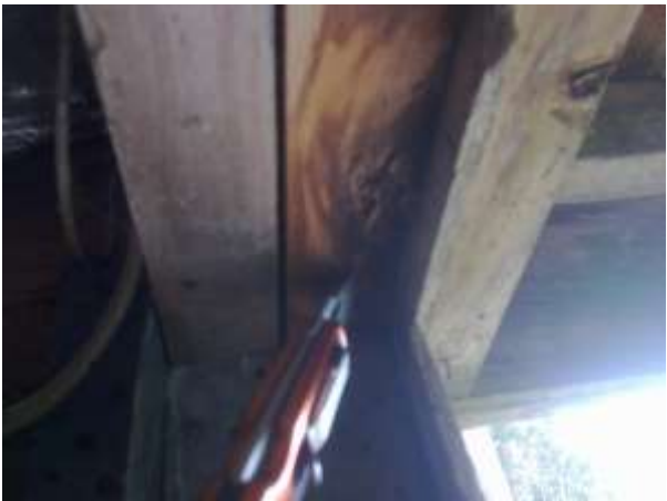
38. The sub floor space. This is a wet & decayed boundary joist on the East wall of the building.
