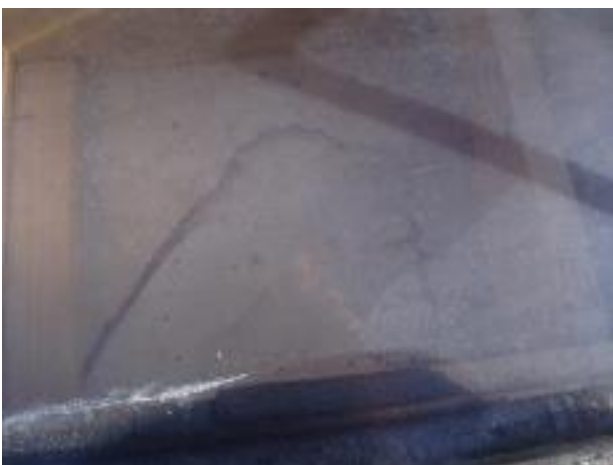
16. Waterstaining is visible on the gib board ceiling of the ensuite bathroom under the skylight. The leak is probably coming from the disused flue.
