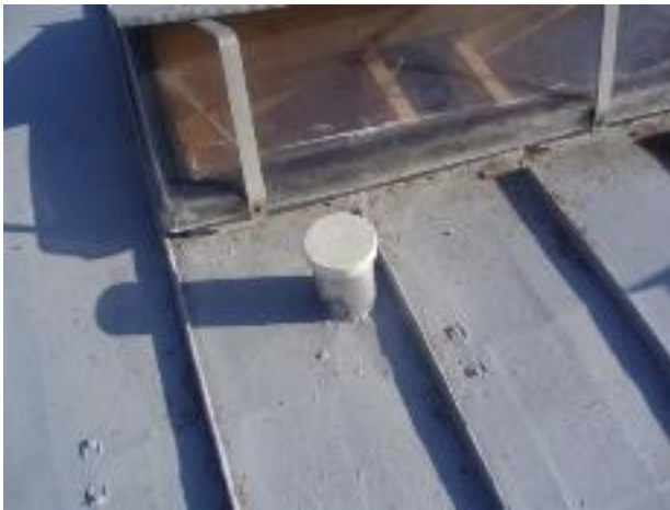
18. The roof has a lot of penetrations that appear to be superfluous.
