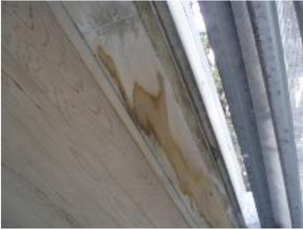
25. This waterstaining to the cedar soffit under the hidden gutter on the North wall is evidence of leaking.
