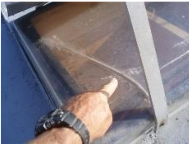
15. A broken skylight. This should be replaced ASAP.
