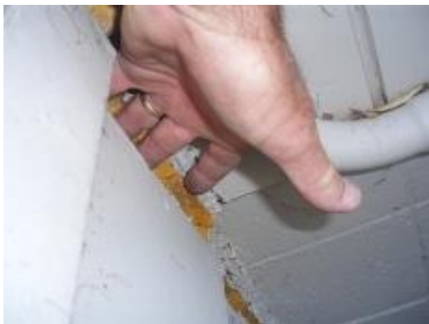
9. The concrete floor of the cupboard off the garage has settled causing this gap to open up.
