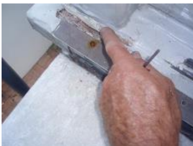
26. Water damage & corrosion is visible all along the base of the North wall.
