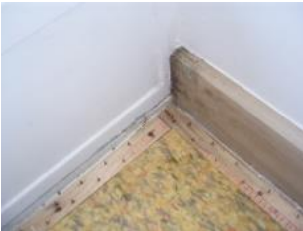
31. The same thing is visible on the skirting board directly below it. Again probably due to the condensation on the joinery unit. I received slightly elevated moisture readings in this location.
