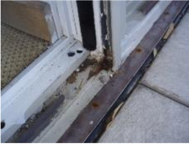
29. Another view of the door track of the North wall. Note the corrosion.
