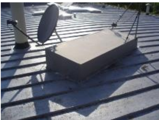
20. The roof has lots of penetrations & junctions. This is always a maintenance hassle on an old flat roof.
