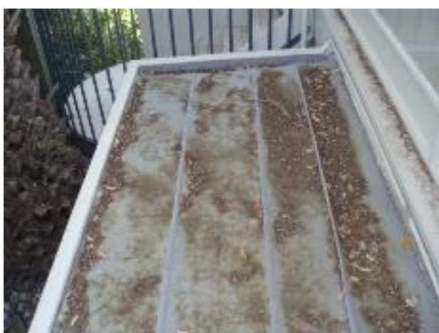
11. There is a lot of debris on the covered roof. It appears to leak & the gutter dropper (downpipe) is very small.
