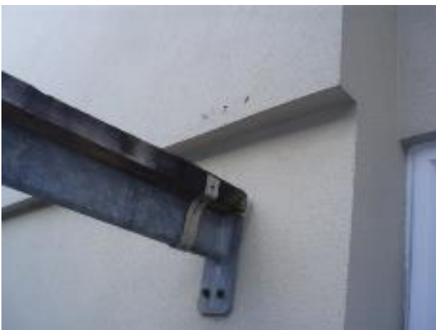
32. Water ingress likely occurs where this gate structure is bolted to the EIFS cladding. Also note the holes drilled in the cladding above the gate structure. They are not stopped up.
