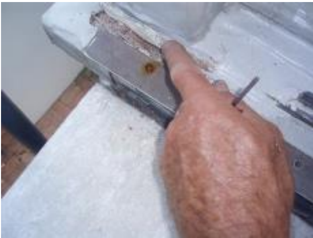
26. Water damage & corrosion is visible all along the base of the North wall.
