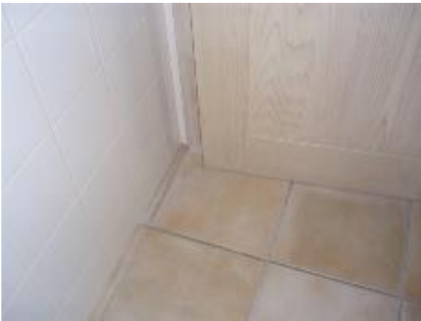
46. The toilet door binds on the floor, I think due to substrate movement.
