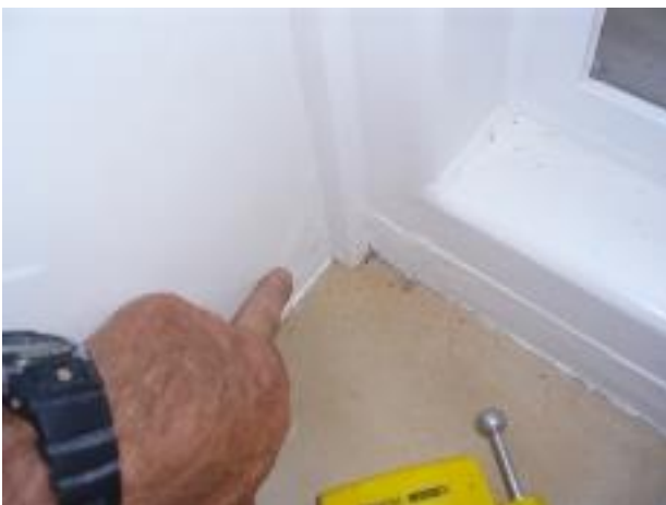
48. Water damage is visible on the gipboard wall in the entry lobby. The water ingress here may well stem from the steel portal highlighted in photo 2 & 3.
