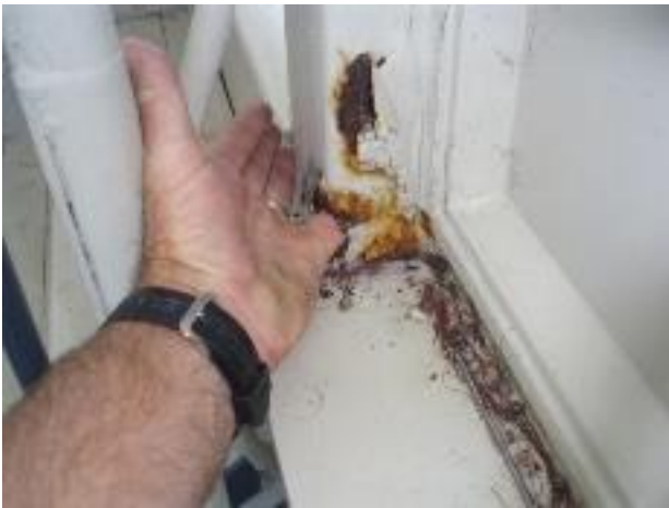
14. This shows severe corrosion of the SHS portal on the NW corner. You can see I have pushed my finger through the rust.
