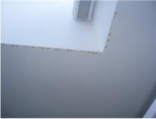
45. The discoloration around the edge of the skylight is caused by condensation / leaking.
