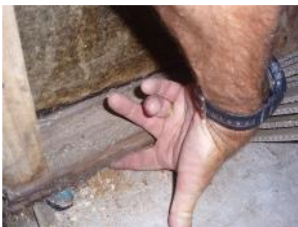
42. The bottom plate of the cupboard is severely decayed.
