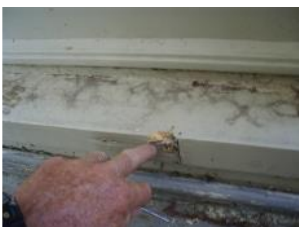
12. A decayed window sill on the Western wall of the lounge.
