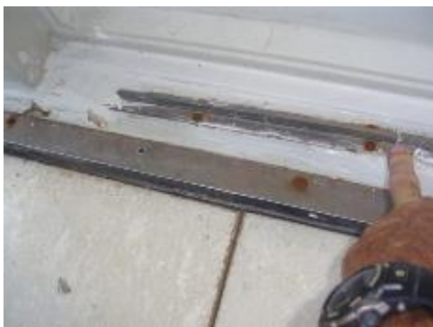
27. I took this photo to show that this area of the door track looked to be in poor condition....
