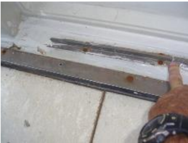
27. I took this photo to show that this area of the door track looked to be in poor condition....
