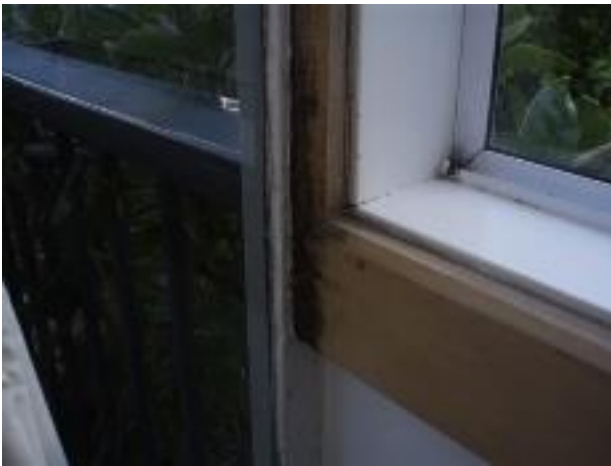
30. In the NE corner of the master bedroom the architrave of the window is discolored & moldy probably due to condensation around the steel window frame on the North wall.
