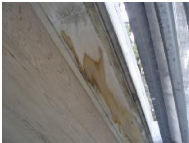
25. This waterstaining to the cedar soffit under the hidden gutter on the North wall is evidence of leaking.
