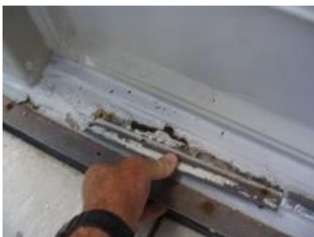
28...and a little later during the inspection I stood on it & it broke away.
