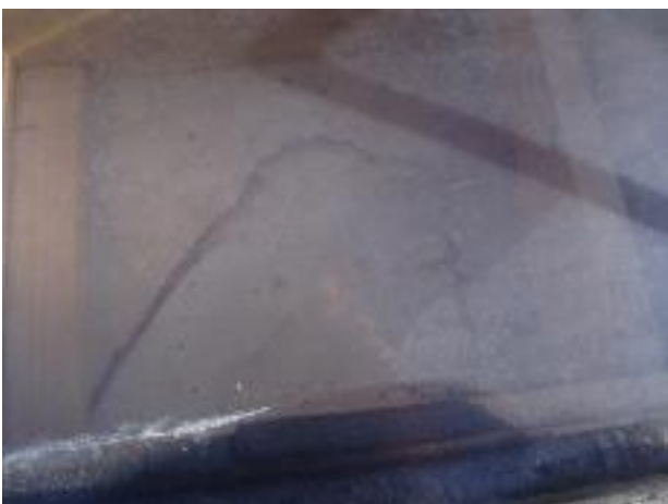
16. Waterstaining is visible on the gib board ceiling of the ensuite bathroom under the skylight. The leak is probably coming from the disused flue.
