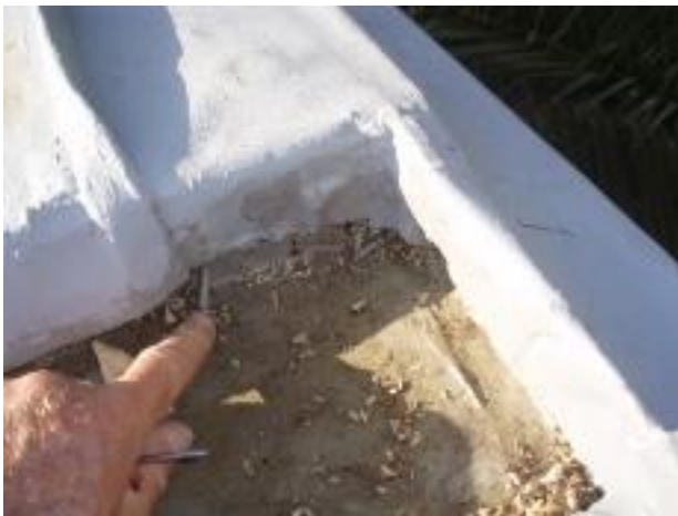
19. The entire roof has been covered with a paint on membrane but not a lot of attention was paid to detail & prep work. As an example I am pointing to a screw that was lying loose in the guttering & simply painted over.
