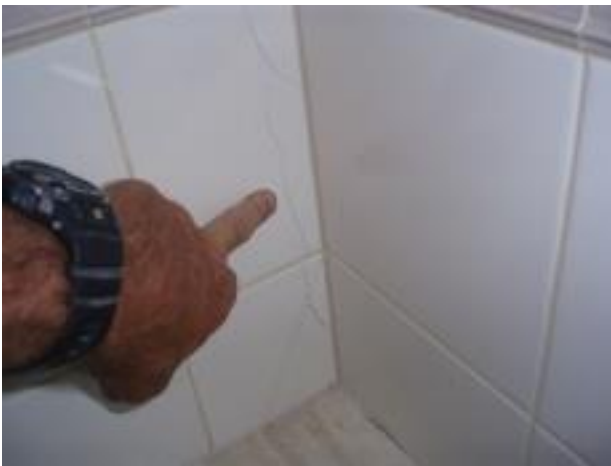
47. These cracked tiles, also in the bathroom, are probably also due to substrate movement.
