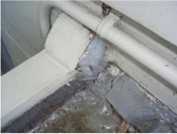
13. This junction of the cupboard roof to the cladding is not weathertight.
