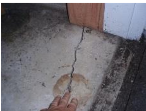
10. This shows the crack in the concrete floor. The floor has slumped noticeably.
