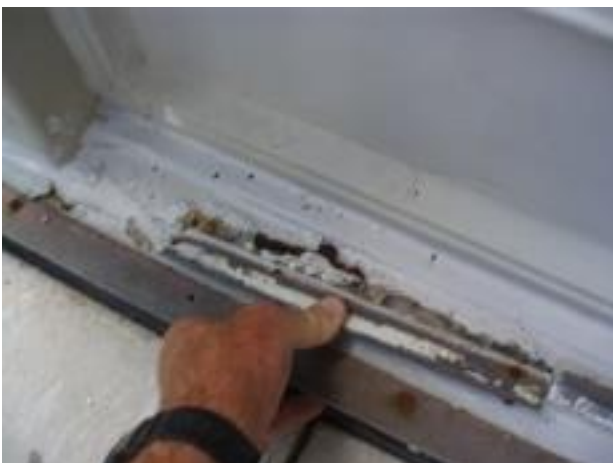
28...and a little later during the inspection I stood on it & it broke away.
