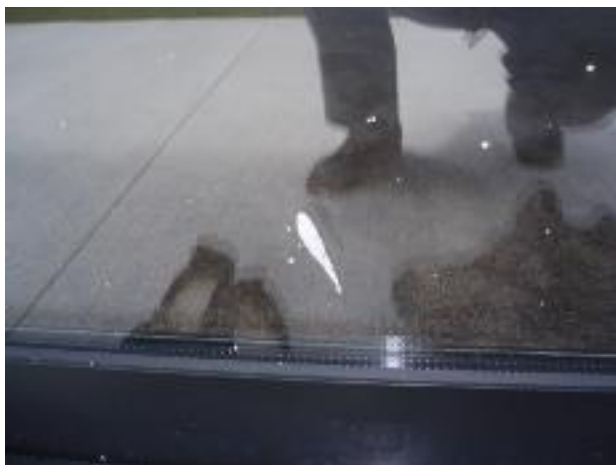
13. This shows concrete splatter on a window & on the aluminium joinery unit. Again there are many examples of mortar & concrete splatter on the joinery units.
