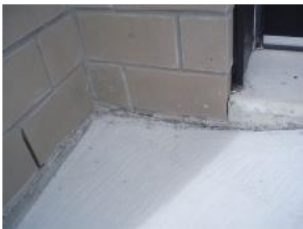
15. Another example of the very poor finish quality of the exterior pavement.
