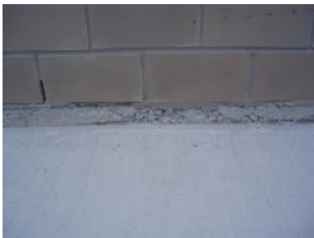
14. The concrete exterior pavement is a very untidy & unprofessional job.
