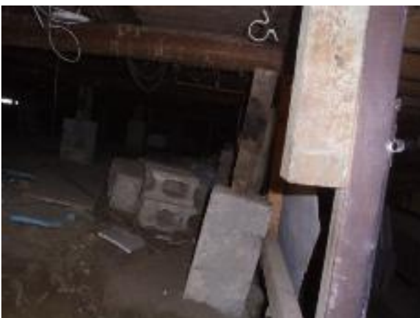
36. This shows a concrete pile that supports a timber jackstud. It has been undermined & has rotated to a significant degree. This should be considered unsafe.
