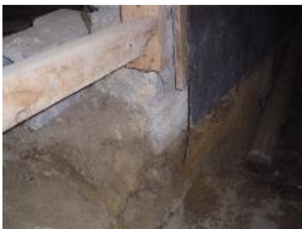
37. Another undermined pile.
