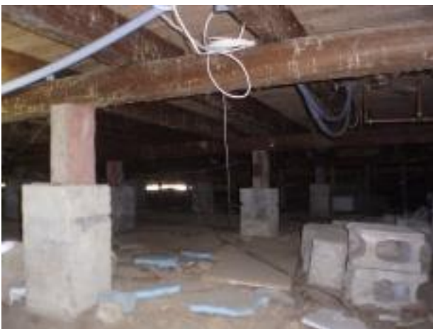
35. The subfloor structure looks to be in generally good condition given its age however sign of borer is present so it requires fumigating. The floor is not insulated. Also some areas have been excavated & the piles undermined. These areas need attention i.e. the undermined piles need to be re-stabilized.
